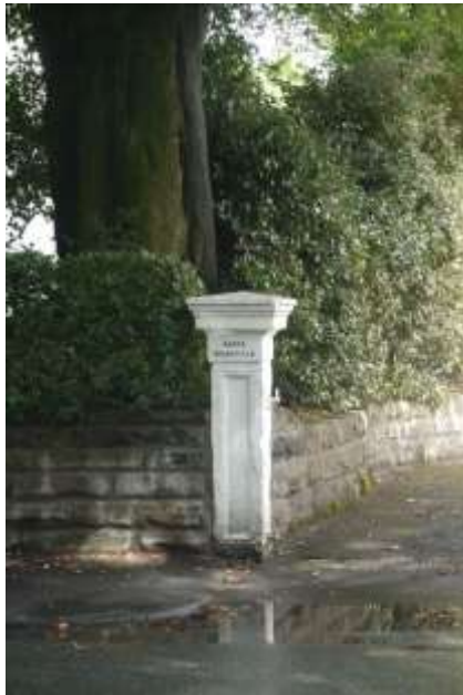
Original gate pier to North Woodville. This has been painted and is showing signs of erosion due to low level water damage.
