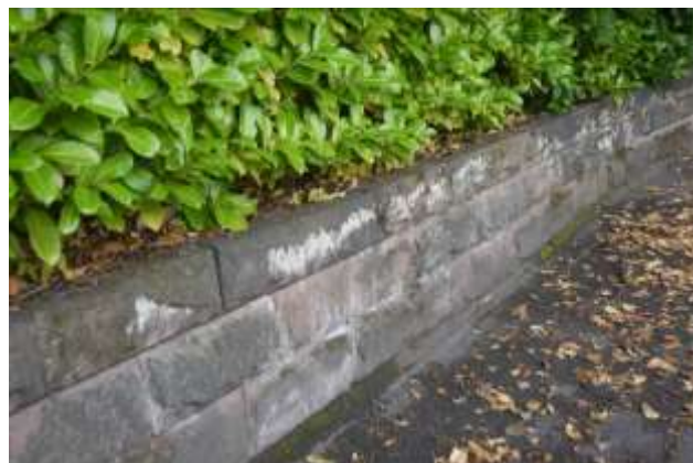
Low stone boundary wall with laurel planting above in Character Zone A
