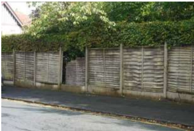
Timber panel fencing in Character Zone A that is inappropriate in style and in a poor condition
